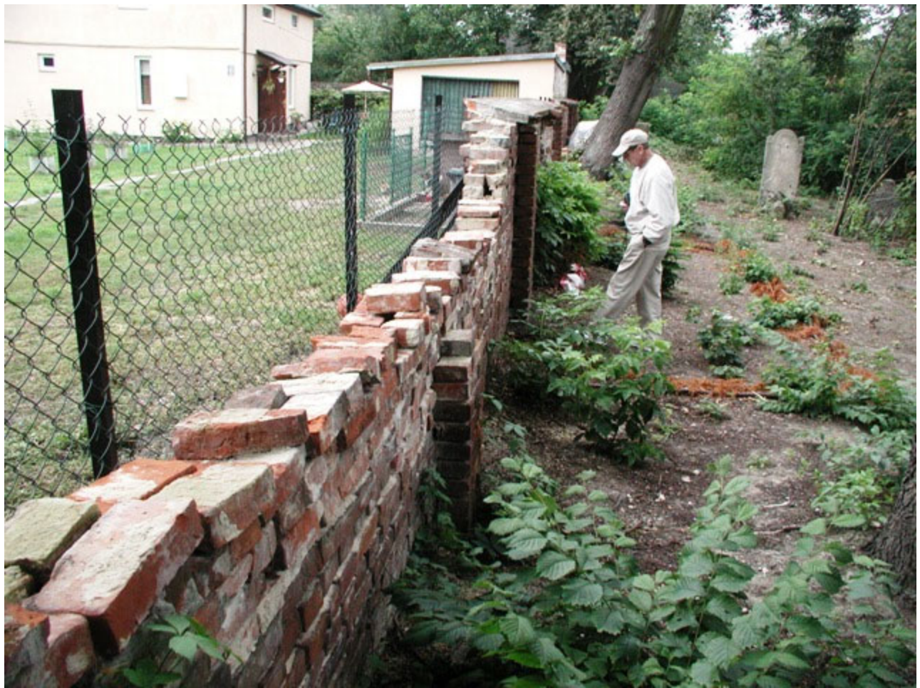
Broken segment of wall September 2007.
