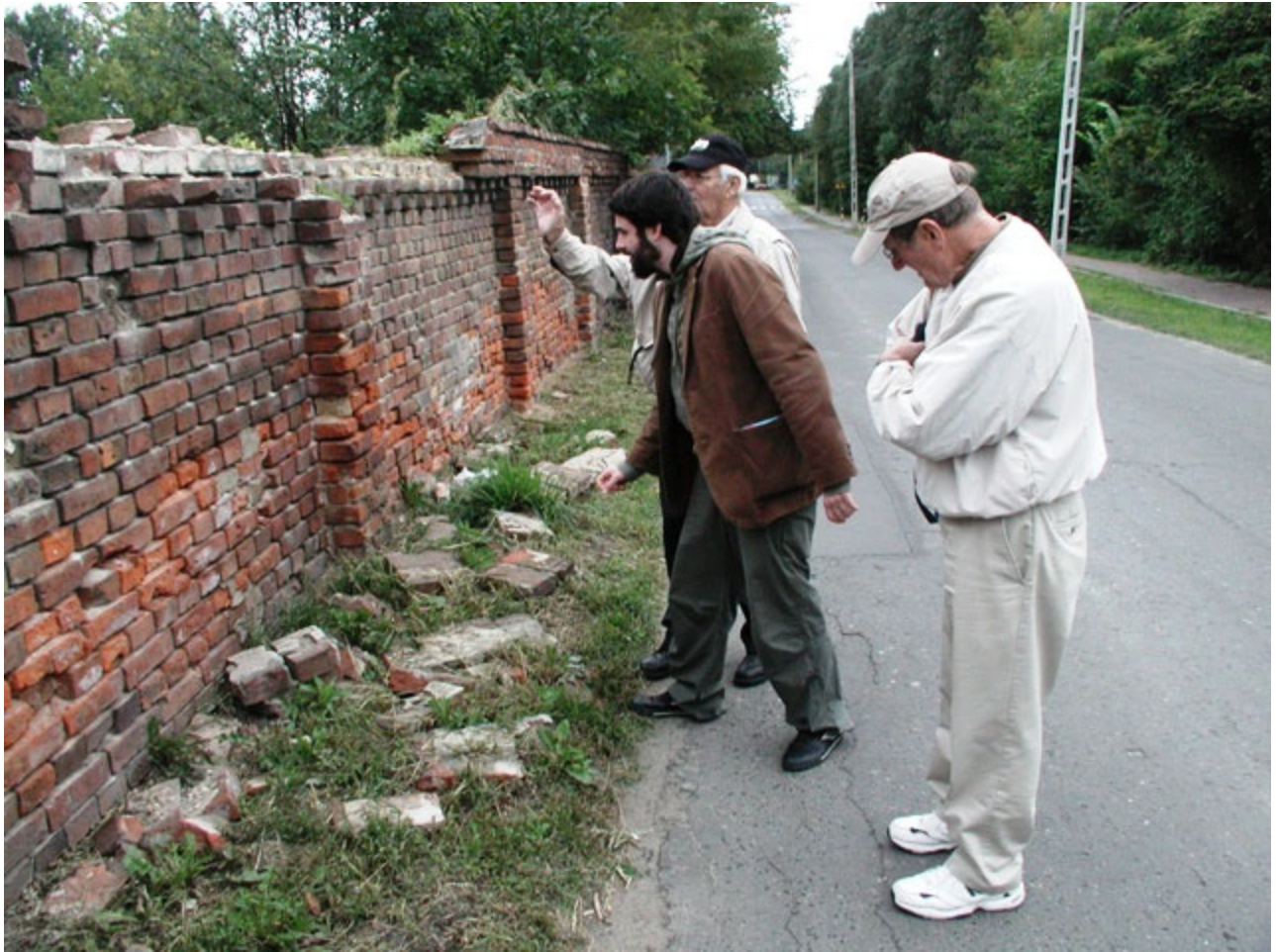
Condition of wall around Pruszkow Jewish Cemetery September 2007 (along main road).
